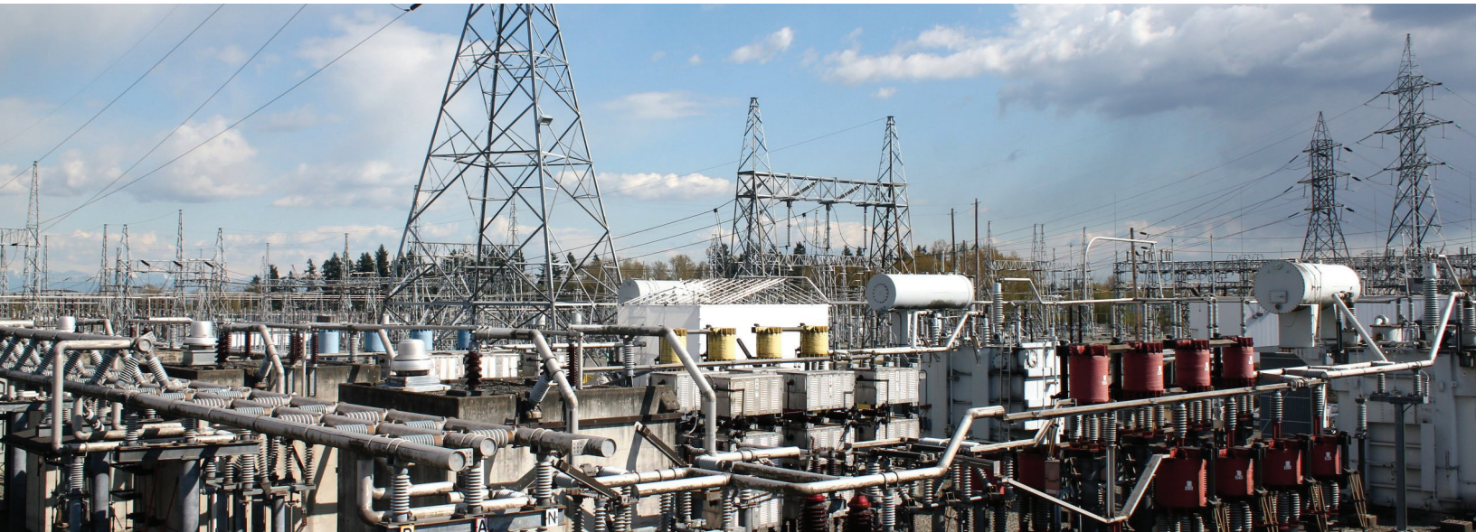
Largest grid-fed high power test facility in North America
