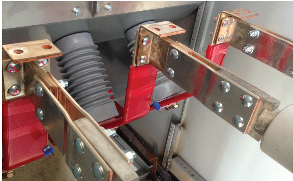
Metal-clad switchgear temperature rise
