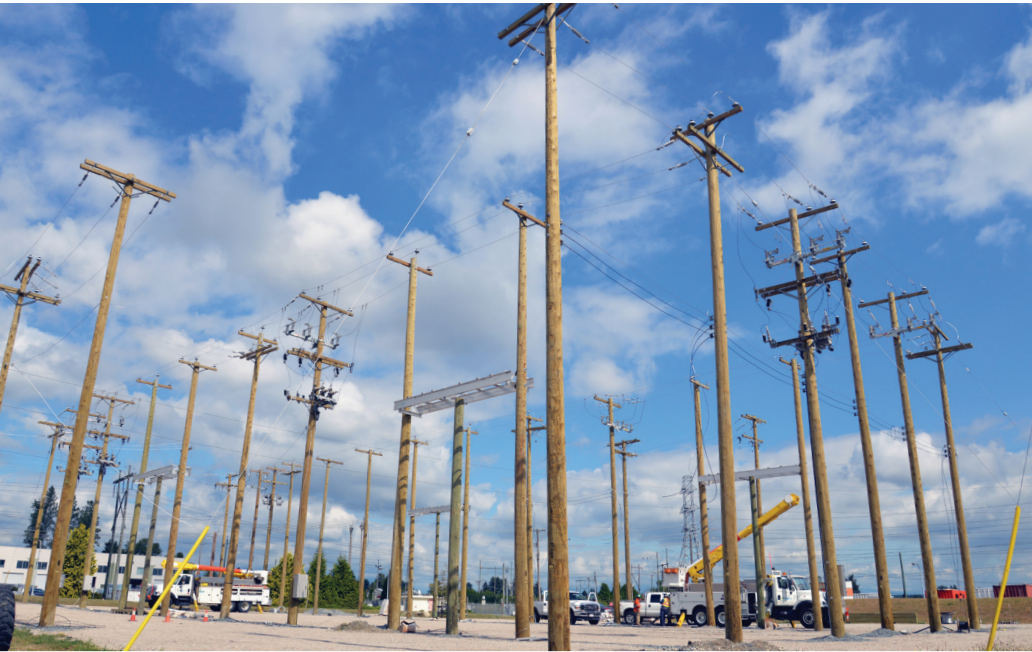
Distribution Automation and Optimization Test Centre
