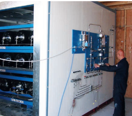
'Fast Fill' hydrogen fueling
