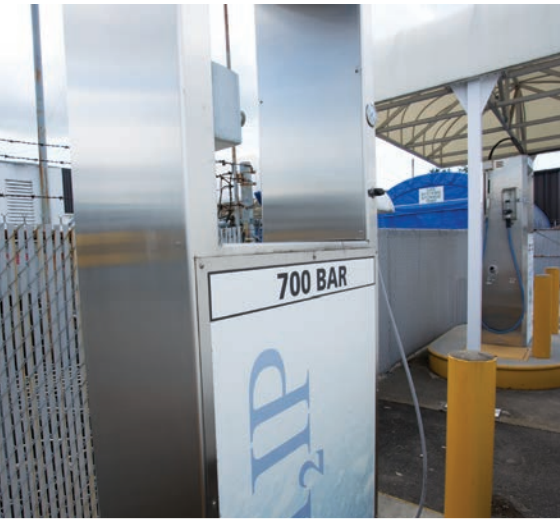
World's first 700 bar hydrogen station
