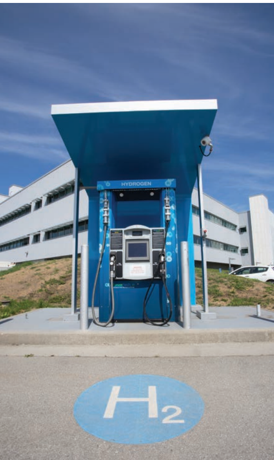
700 bar station located at Powertech
