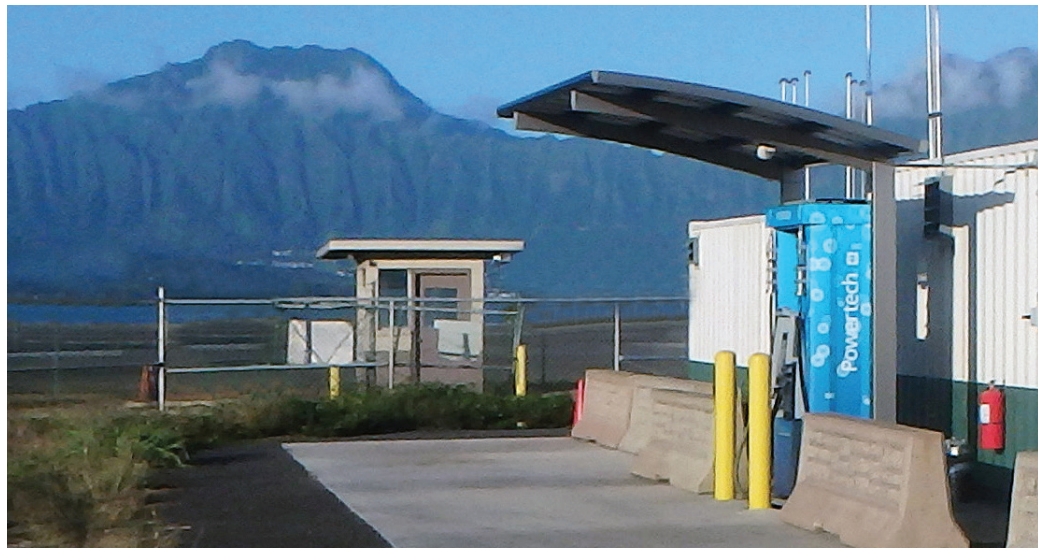
Hawaii 700 bar fueling station
